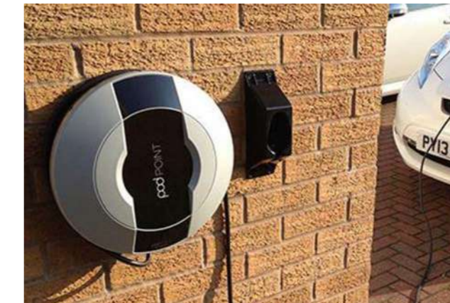
Figure 67: Home electric vehicles charging point
